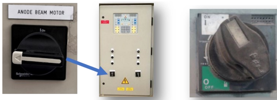
Figure 4. Left: Example of an anode beam motor switch, Middle: Example of a pot control cabinet, Right: Example of an anode beam motor switch. The type of switch differs by the smelter.
