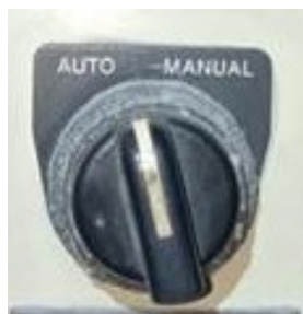
Figure 6. Auto/manual switch present on the pot control cabinet.
